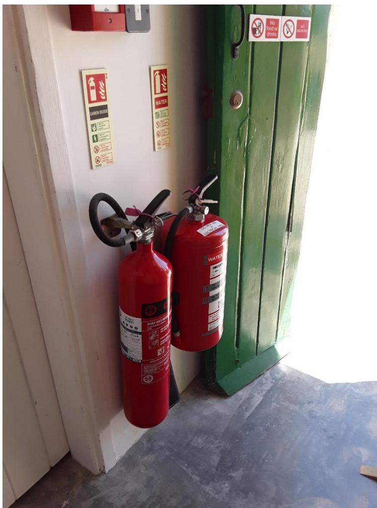
Fire extinguishers placed exactly at each entrance/exit
