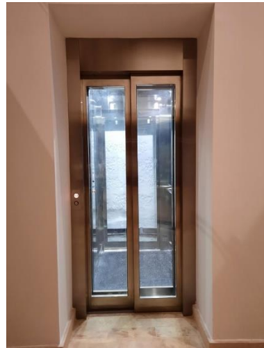
Figure 9: Elevator found in first floor galleries
