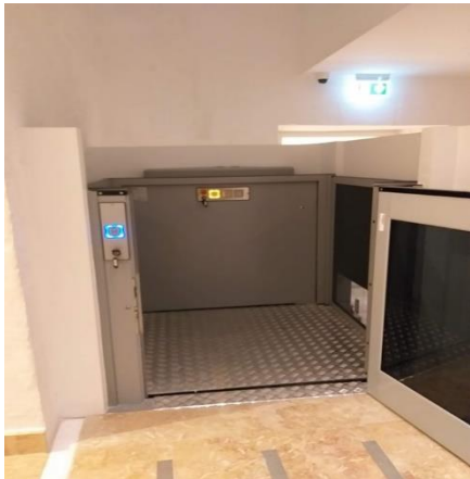
Figure 8 disabled elevator found inside the first-floor galleries.
